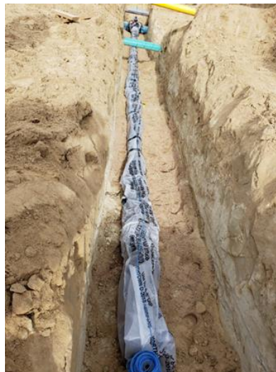
Verification of saddle valve, bedding, pipe wrap, tracer wire and joint constraints (courtesy of Steve Iacino, FFFPD).
