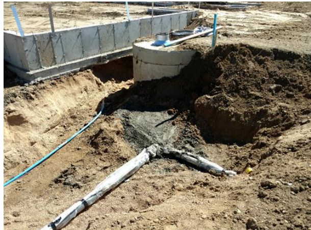
Concrete thrust block installed between underground supply line and undisturbed soil (courtesy of Steve Iacino, FFFPD).
