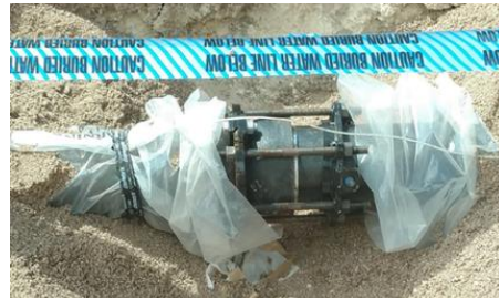
“Jeeping”-using corrosion retarding material to protect underground supply lines (courtesy of Steve Iacino, FFFPD).
